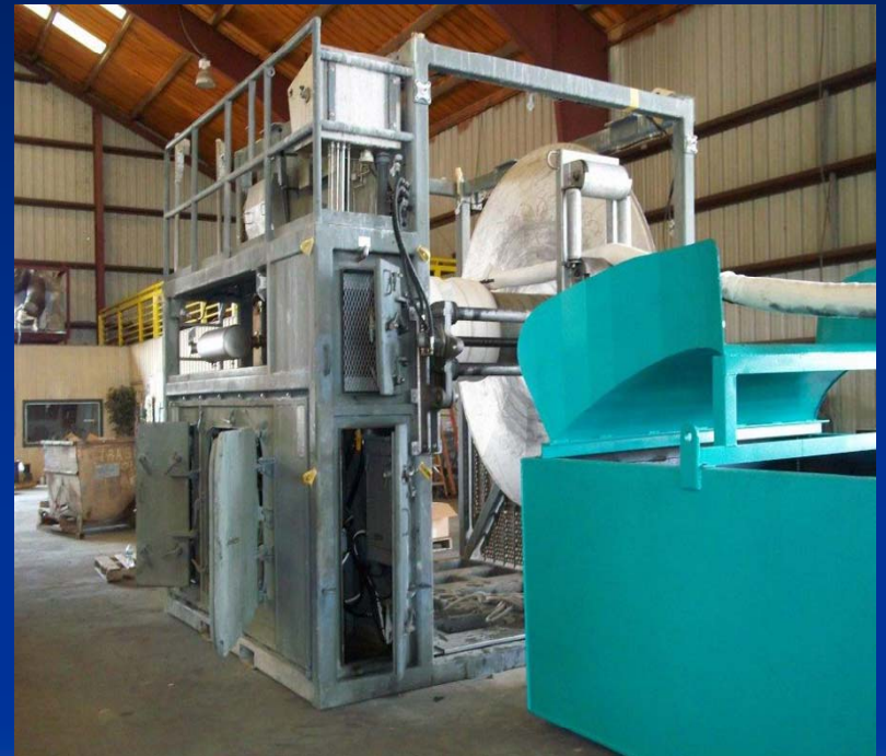
OIL RECOVERY SYSTEM
